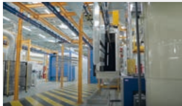
Automatic powder coating line
