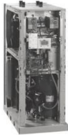
Access to control panel
